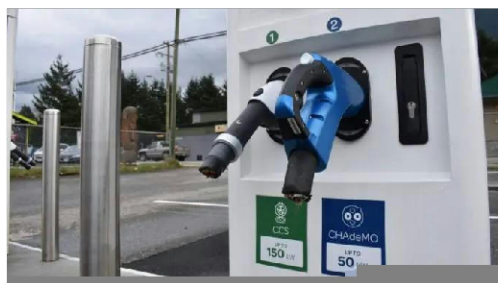
Electric vehicle charging station with severed cables.
