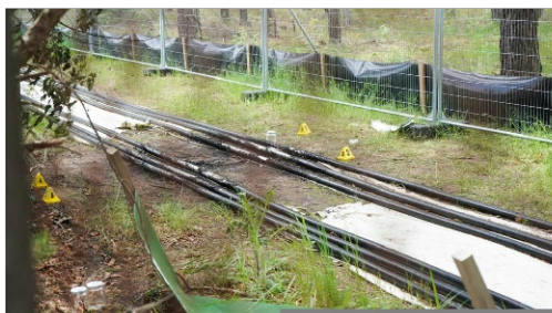
Six high-voltage cables supplying power to the site of a Tesla “gigafactory” were torched near Berlin, Germany in May 2021. Translated from the communique 24 : “Our fire opposes the lie of the ecological car”.
